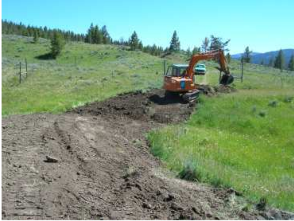
Photo 13. Decommissioning - This photo in T9S R3E S1 was taken on 7/27/05. A culvert was removed and stream banks restored to pre-road channel geometry. The area was then seeded and hydro mulched. Revegetation response is expected to be robust. The treatment is designed to eliminate the road as sediment source and avoid a long term potential sediment source if the culvert fails. The road decommissioning work on Gallatin NF lands during 2002-2005 has removed 55 culverts in the Taylor Fork watershed.
