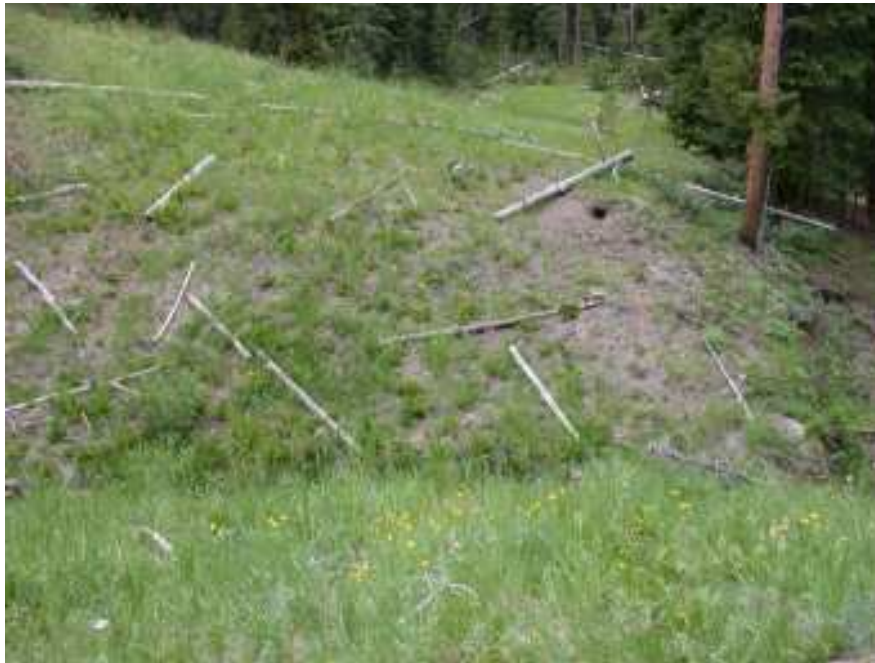
Photo 7. East Fork FK Cache Ck Road. The road surface was ripped, seeded, and drained. Logs were placed on cutbank slope to catch sediment and stabilize the slope.
